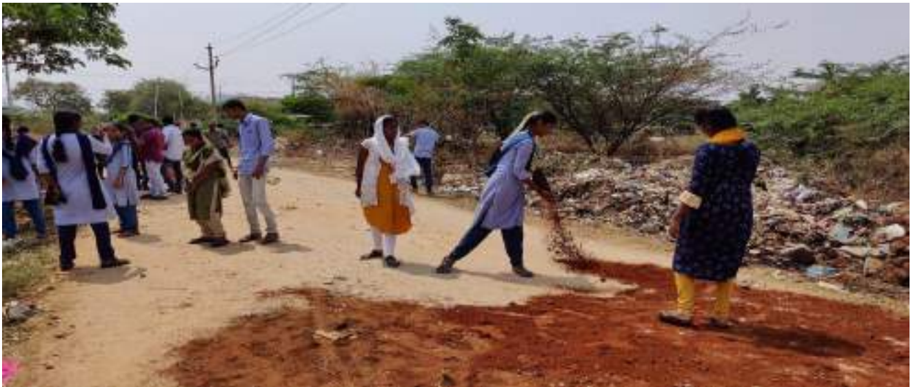
Formation of Road from SC Colony to Yerraguntla Palli by NSS Volunteers
